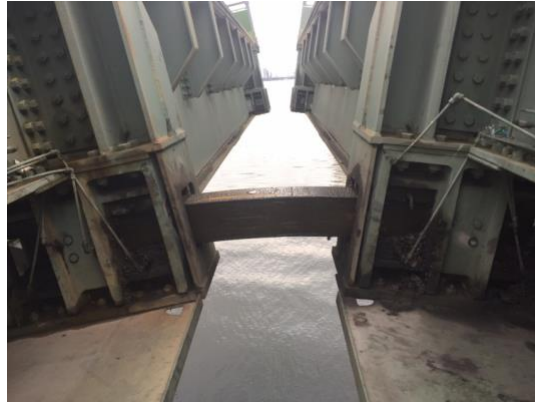
Figure 15 - Lock bar damage on Brickell Avenue Bridge in Miami after lock limit switch failure – via FDI Services
